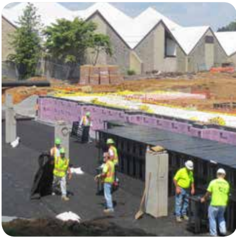
Water Detention Systems
